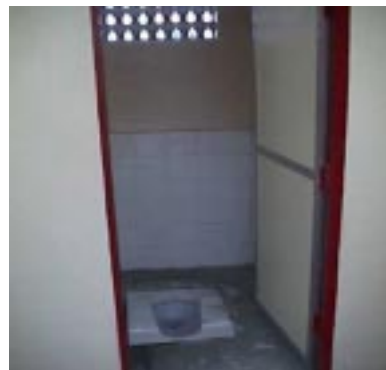
One new stall at Bharat Nagar, showing the floor and wall tiling, and the bison board doors
