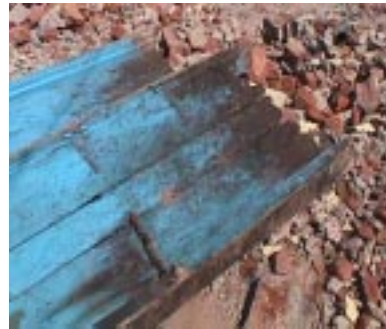
During demolitions at Sangam Wadi: you can see the rotten state of the old wooden doors.
