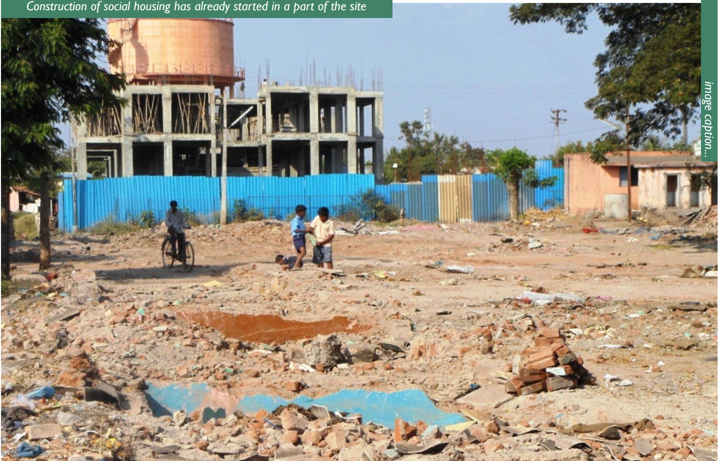
Construction of social housing has already started in a part of the site
