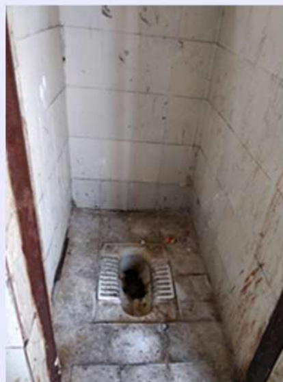
Condition of CTB in Anand nagar
