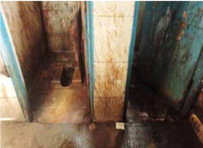
A “poor” condition toilet in a community toilet block that is used everyday by women in Pune
