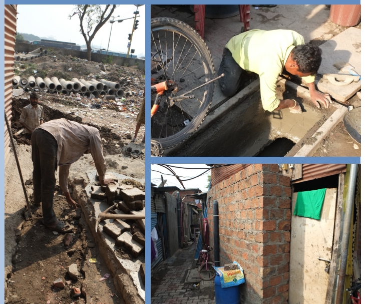
The mason's work covers the whole construction process, from toilet seat, building to tiles, door setting, and connection to drainage line. Often, it also included the construction of a new front wall.
