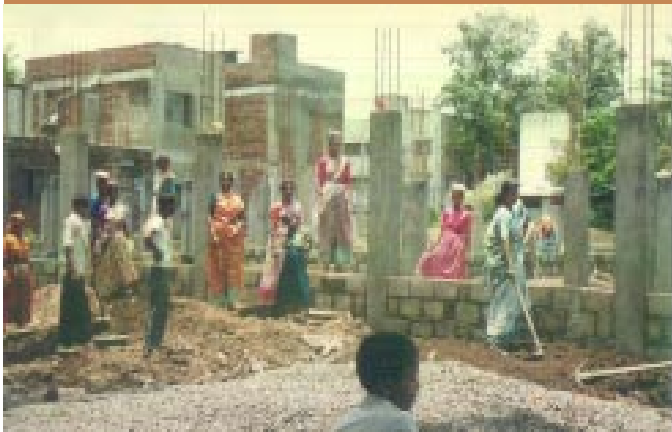
BELOW: working together on site; putting up the beams; tamping; training other communities RIGHT: laying the laadis on the beams; view across the courtyard of the completed building
