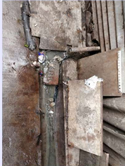
Gutter opposite their house
